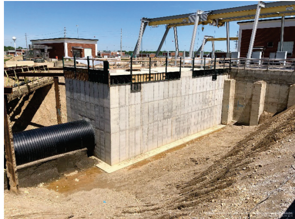
Photograph of the construction of the CEPT Dechlorination Structure at the Southerly Wastewater Treatment Plant.
