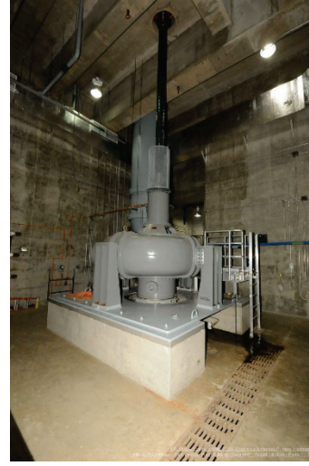
Photograph of a new Raw Water Sewage Pump at the Southerly Wastewater Treatment Plant.
