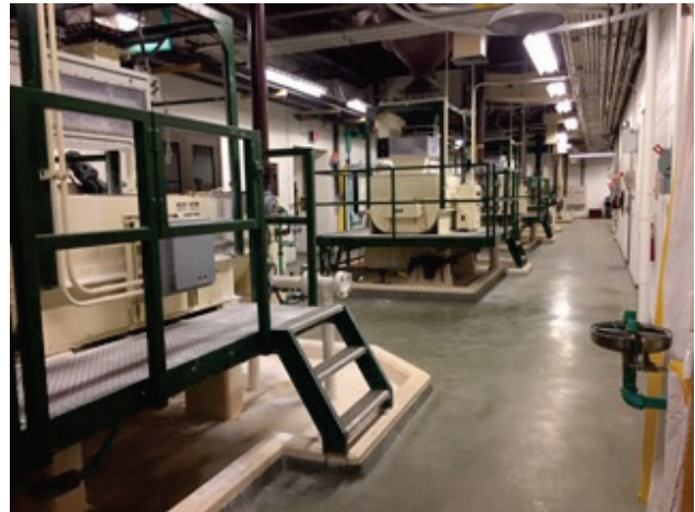
Existing Lime Slakers at PAWP. New Slakers & Feeders will increase the reliability of the water supply system.
