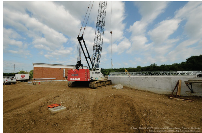
Photograph of the construction of the CEPT Chemical Building and Clarifier at the Southerly Wastewater Treatment Plant.
