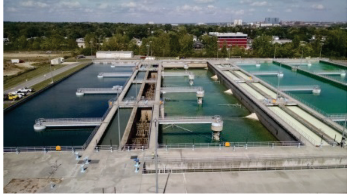
Existing treatment basins and clarifier equipment will be replaced under this project.
