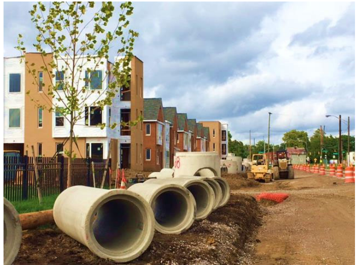
Photograph of the newly added housing units in the Poindexter Village area, currently under construction.
