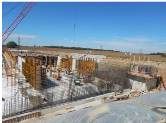
Installation of a new clearwell at PAWP. This will increase the reliability of the water supply system.
