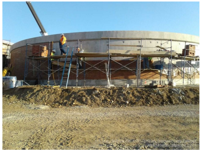
Photograph of the construction of the new Gravity Thickener at the Southerly Wastewater Treatment Plant.
