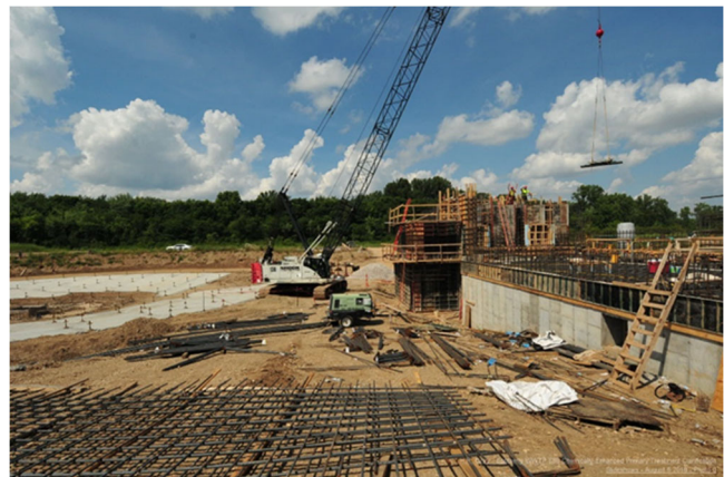
Photograph of the construction of a CEPT Chemical Building and Primary Clarifier at the Southerly Wastewater Treatment Plant.
