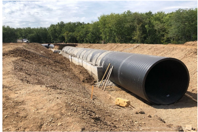
Photograph of the construction of the CEPT effluent pipeline at the Southerly Wastewater Treatment Plant.
