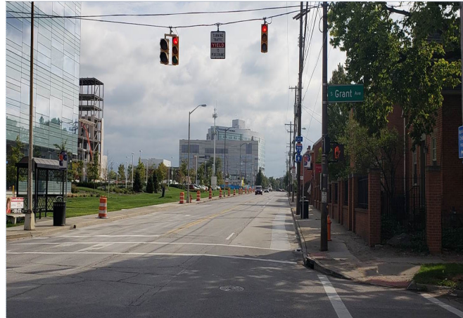
Preparing to deploy orange barrels on Livingston Avenue so project work can begin.
