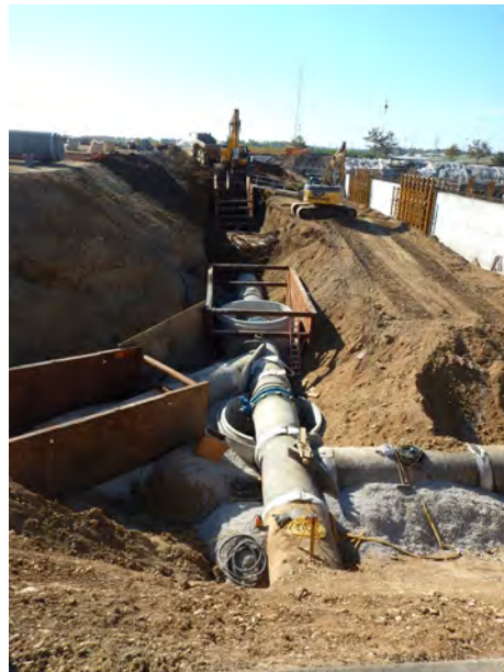
Installation of a new clearwell at PAWP. This will increase the reliability of the water supply system.
