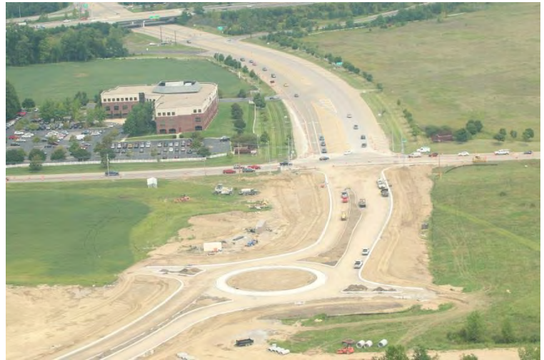
Aerial photograph of construction in progress of a new round-about for the N. Hamilton Road “S” curve at State Route 161.
