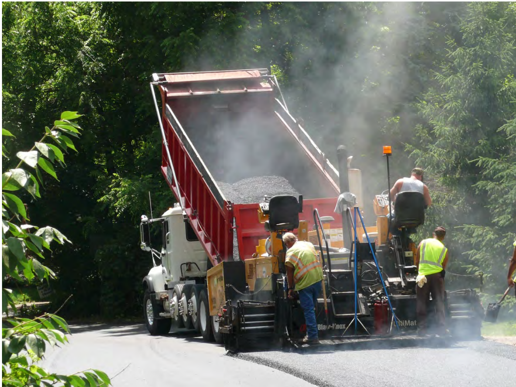
Road being resurfaced with new asphalt as a continued part of the city's resurfacing commitment.
