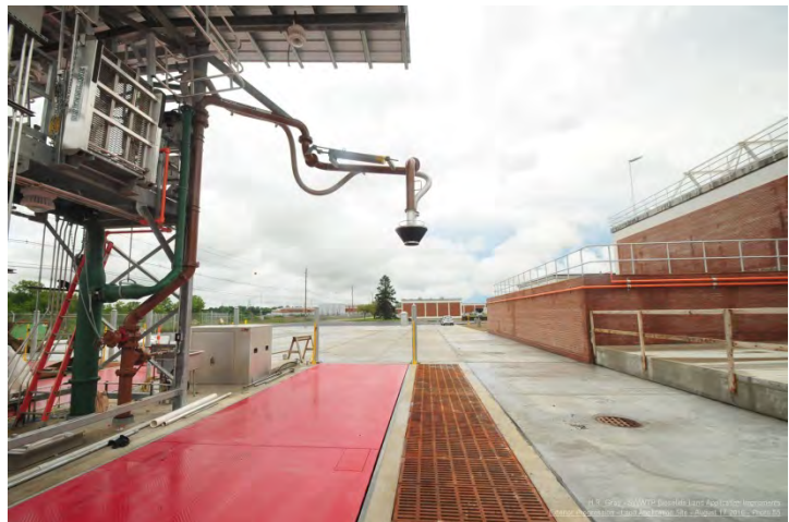
Photograph of the Truck load-out portion of the Southerly Waste Water Treatment Plant.
