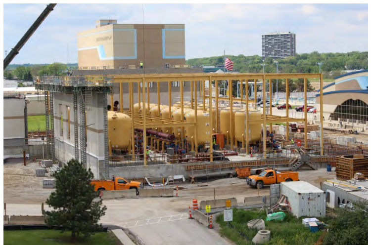
Construction on the new ion exchange treatment portion of the DRWP Capacity Increase.
