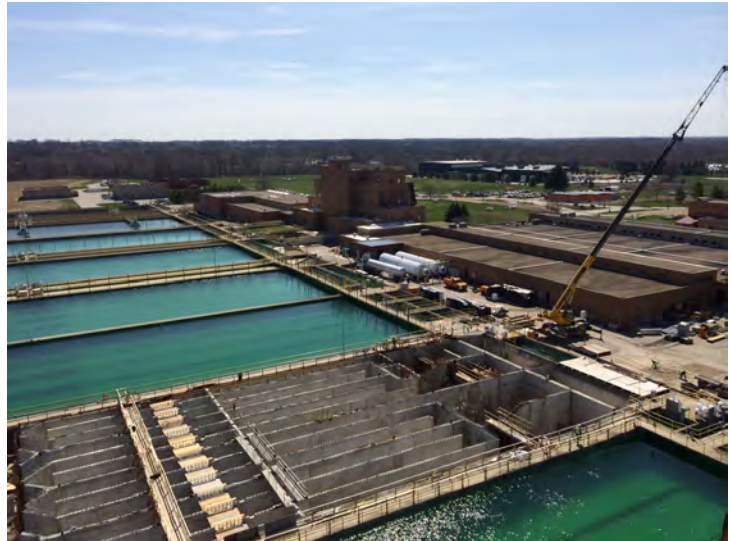
Construction of a portion of the water treatment improvements located at HCWP.
