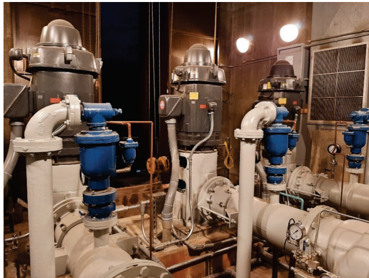
View of the PAWP CW104 new motors for the three vertical turbine pumps
