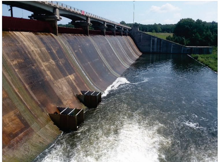
View of Hoover Dam spillway showing the temporary cascade aerators installed under this project
