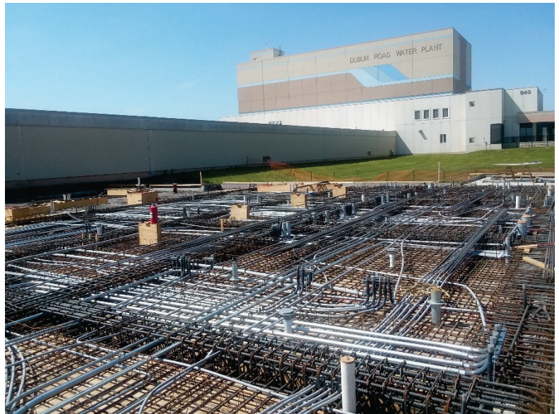
Installation of rebar and conduit in the DRWP UV Facility's first floor slab
