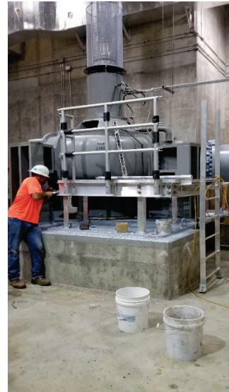
Installation of the Access Platform for RSP 1 at the Southerly Wastewater Treatment Plant.
