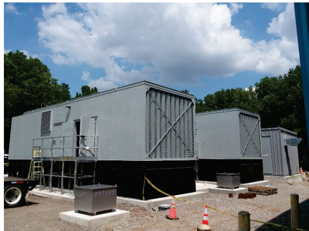
View of the DRWP's two new standby generators and switchgear.
