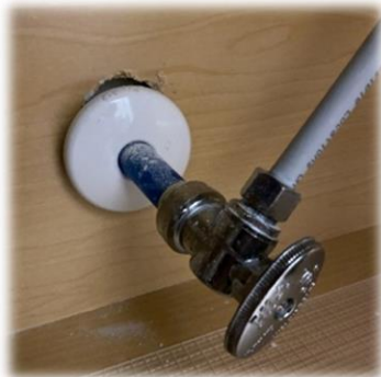
These quarter turn valves are notorious for failing and seizing
