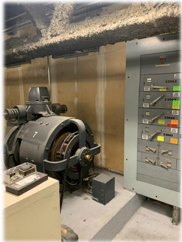
This is a traction elevator system located at 155 E. Broad Street (PNC Building)
