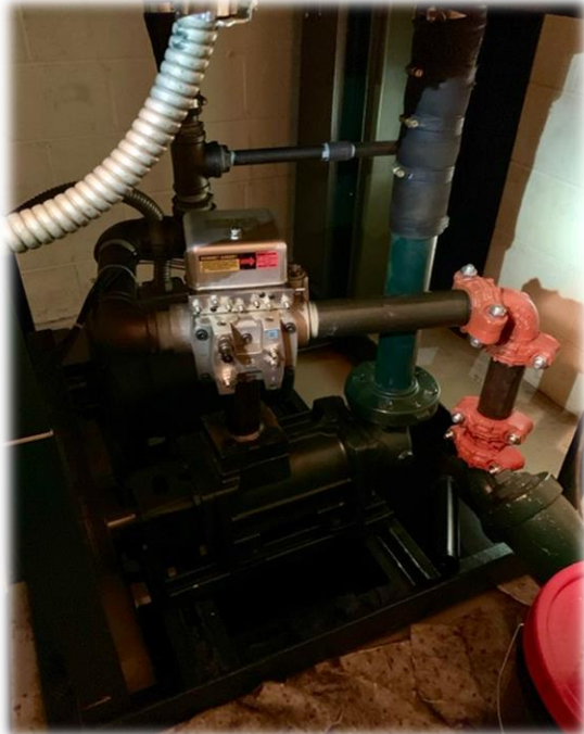
This is the hydraulic pump manifold from 170 E. Town Street
