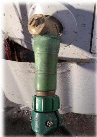
Water thief adapter and utility hose attached to the hot water tank drain
