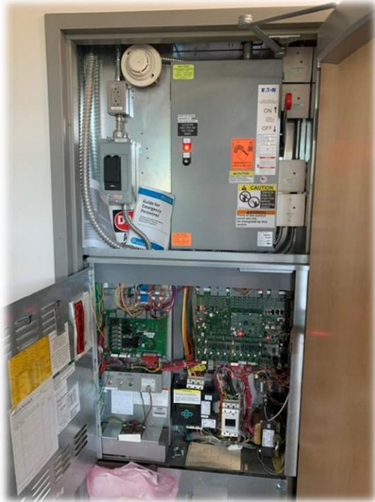
This shows the elevator machine “room” for a hydraulic driven MRL system
