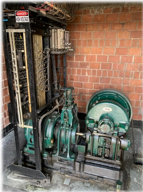
This is an Otis traction elevator system located at 1445 E. Broad Street
