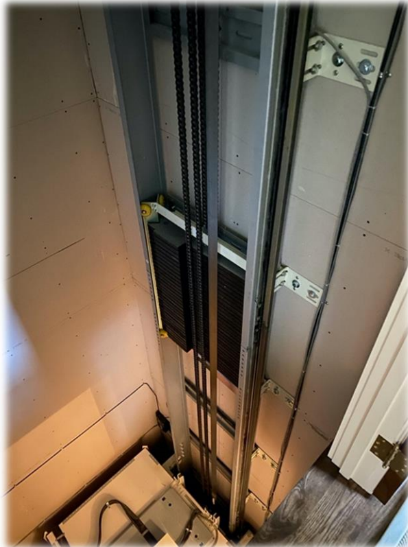
This shows the counterweights, guiderails, and drive belt built within the hoistway of a residential MRL elevator
