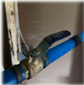
This inline valve's handle is in line with the plumbing, meaning the water is on
