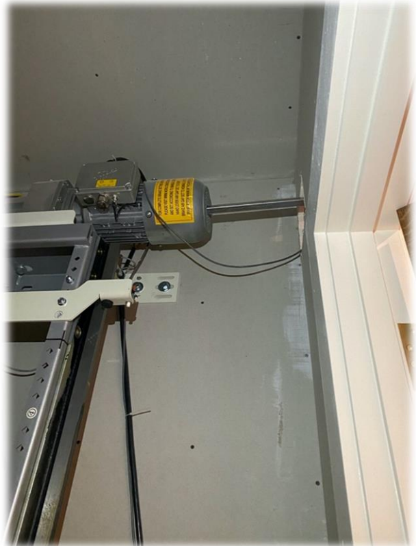
This shows the motor located at the top of the shaft with a metal manual override rod inserted into it. This rod can be used to lower and raise the car by hand
