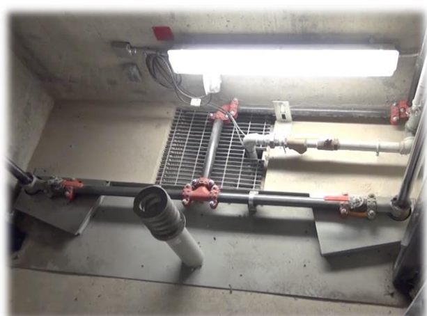
This is the bottom of the elevator shaft of the Training Academy hydraulic evaluator. Pictured is the main plumbing coming in from the reservoir to both multistage lift cylinders
