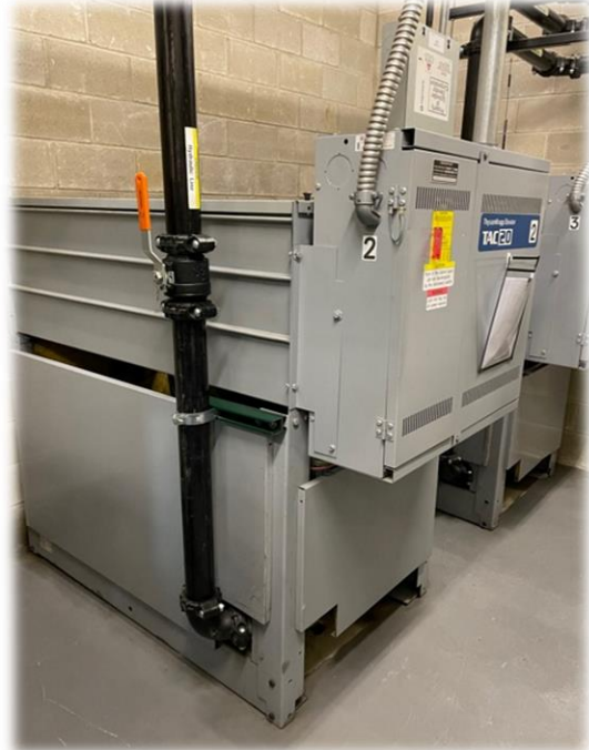
This is the hydraulic equipment room at South Campus Gateway Parking Garage
