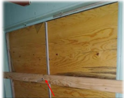
Similar to drop bars, carriage bolts can indicate the plywood is secured from behind. A chainsaw can still defeat this by plunging in past the 2x4.
