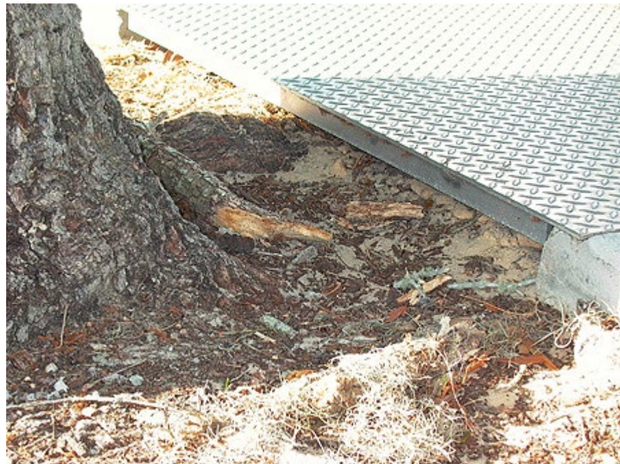
Figure G7. Sidewalk bridging over tree roots. Photo: Edward F. Gilman, Professor, Environmental Horticulture Department, IFAS, University of Florida
