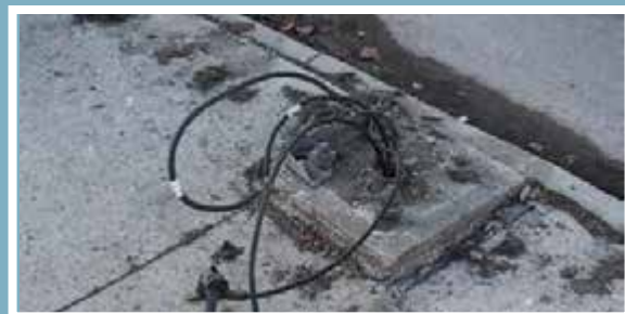
LACK OF PEDESTRIAN-SCALE LIGHTING
