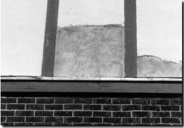
{ PHOTO 8 } Stucco wall being repaired to match existing surface. Note the metal flashing between the stucco wall and the wood horizontal trim board.
