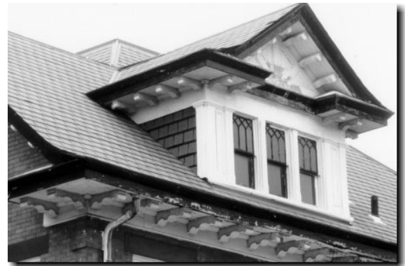
{PHOTO 32} Slate roofing material used as siding. Wood corner boards complete the trim and match the rest of the house.
