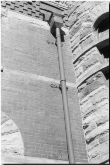
{ PHOTO 27 } Decorative scupper helps collect runoff to the downspout.
