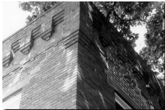
{PHOTO 14} A stepped or corbeled cornice. Note the recent repointing that does not match the existing mortar.
