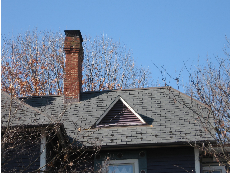
Example of a synthetic slate roof in a Roanoke, Virginia historic district.
