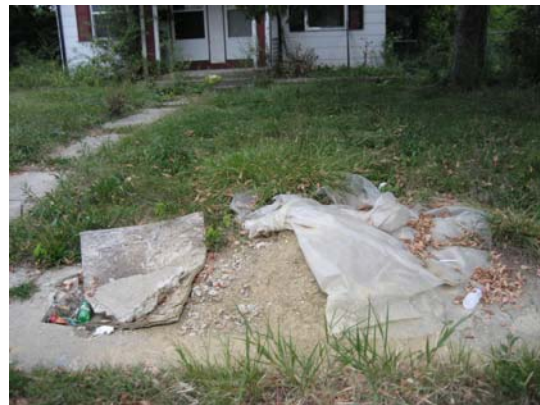
Sidewalk in disrepair and impassable at 1616 Whittier Street.
