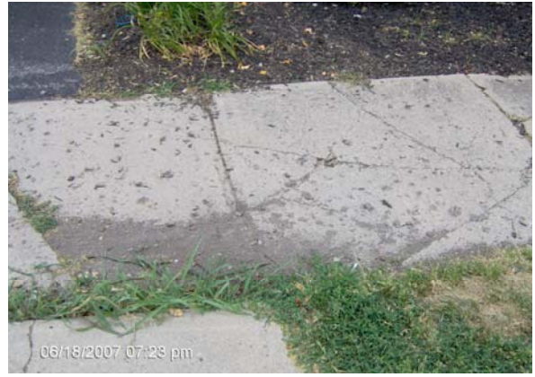
Picture 2. Broken and uneven sidewalks on High Street, west side of the street, between Graceland Shopping Center and Dominion Blvd. (pictured sidewalk is south of Riverview Park Drive)
