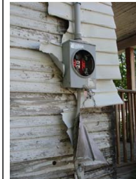
Copper thieves leave exposed electrical.
