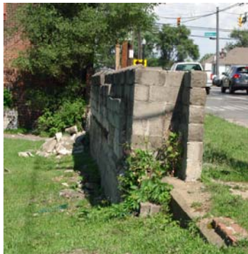
Old building wall is unsafe.
