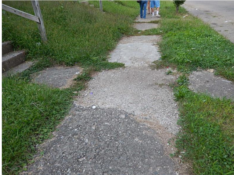
Part of the sidewalk is missing.
